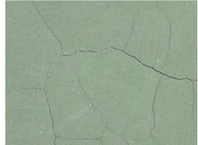
Cracking of subsurface
